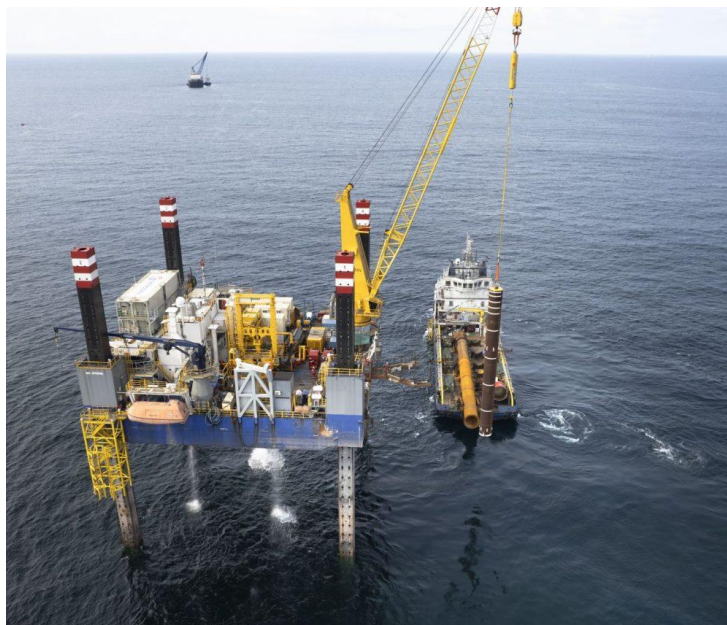
Installation of FLNG mooring system at Eni Congo LNG project; Source: Geocean
